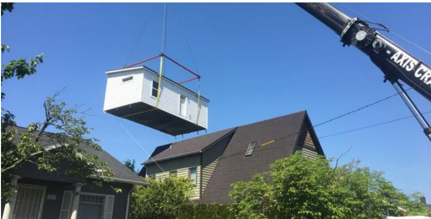
An example of a prefabricated ADU 1 being craned into a residents backyard.
