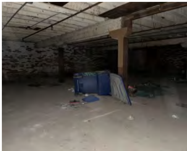
Photo 22 Comments: Basement 1 containing misc debris.
