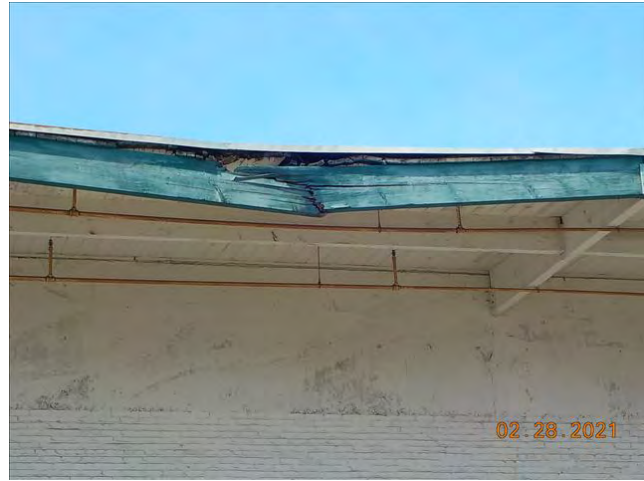
Date: 2/28/2021 9:35:01 AM DAMAGED ROOF AND FASCIA ON H ST. SIDE OF STRUCTURE
