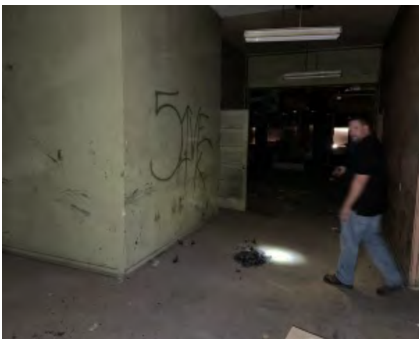
Photo 11 Comments: Southeast end of building looking southeast. Area is split into several rooms.
