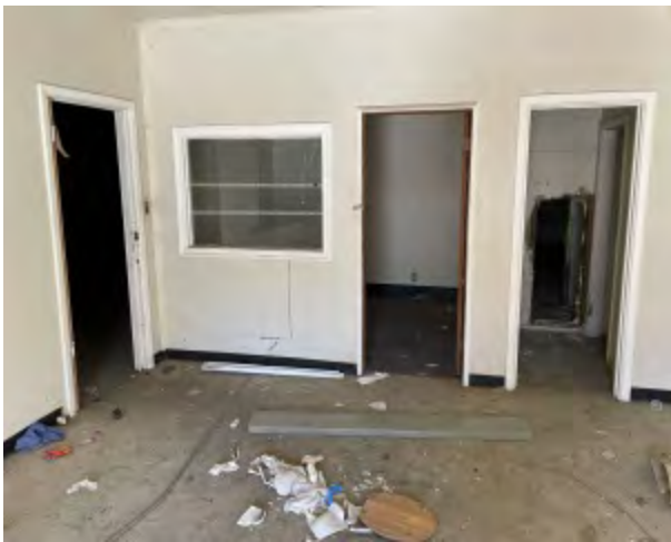
Photo 9 Comments: One of several rooms at middle of building. This is the first room observed upon entering building
