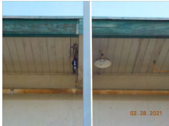
Date: 2/28/2021 9:36:50 AM DAMAGED ROOF ON PARKING LOT SIDE OF STRUCTURE
