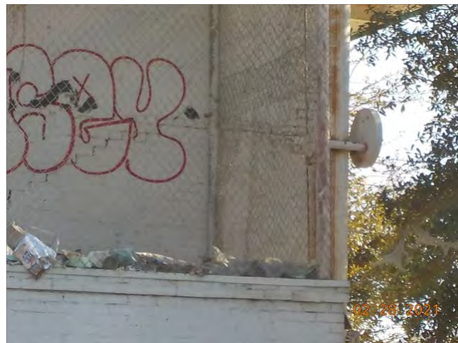
Date: 2/28/2021 9:37:22 AM HOLE IN FENCE, MONO SIDE OF SCTRUCTURE
