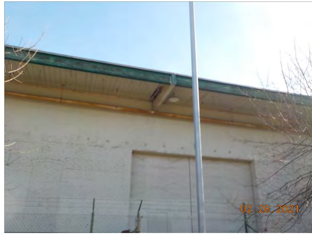
Date: 2/28/2021 9:36:30 AM DAMAGED ROOF ON PARKING LOT SIDE OF STRUCTURE
