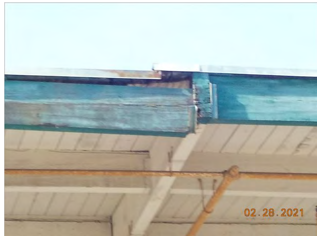
Date: 2/28/2021 9:35:20 AM DAMAGED ROOF AND FASCIA ON H ST. SIDE OF STRUCTURE
