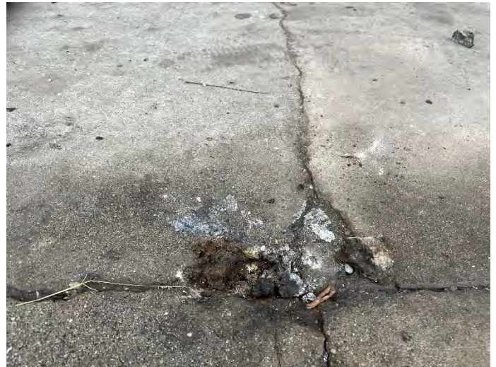
Loading Dock Concrete - Damaged
