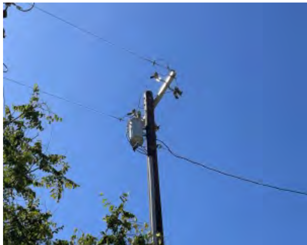
Photo 36 Comments: Single pole mounted transformer located near south corner of building along Mono St.
