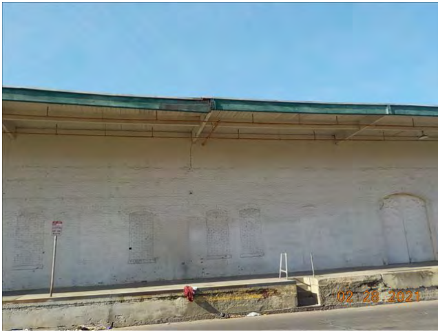
Date: 2/28/2021 9:35:31 AM DAMAGED ROOF AND FASCIA ON H ST. SIDE OF STRUCTURE
