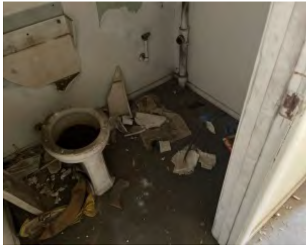
Photo 8 Comments: One of two restrooms located at middle of building. Floor drain observed.
