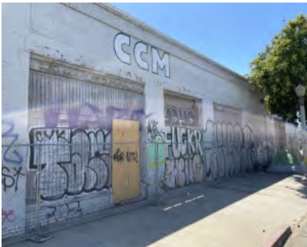
Photo 41 Comments: Strip of buildings located on northeast side of H Street. Buildings are boarded and fenced.
