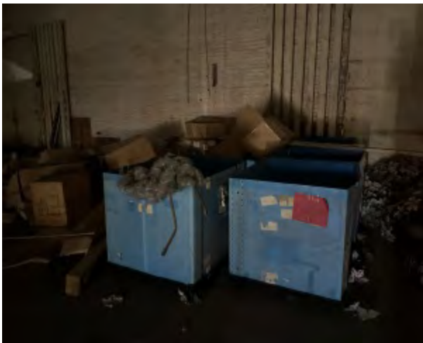
Photo 3 Comments: Northwest end of building. Large bins containing debris and Christmas decor.
