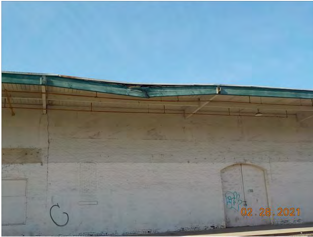
Date: 2/28/2021 9:34:56 AM DAMAGED ROOF AND FASCIA ON H ST. SIDE OF STRUCTURE
