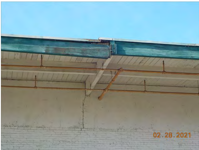
Date: 2/28/2021 9:35:15 AM DAMAGED ROOF AND FASCIA ON H ST. SIDE OF STRUCTURE
