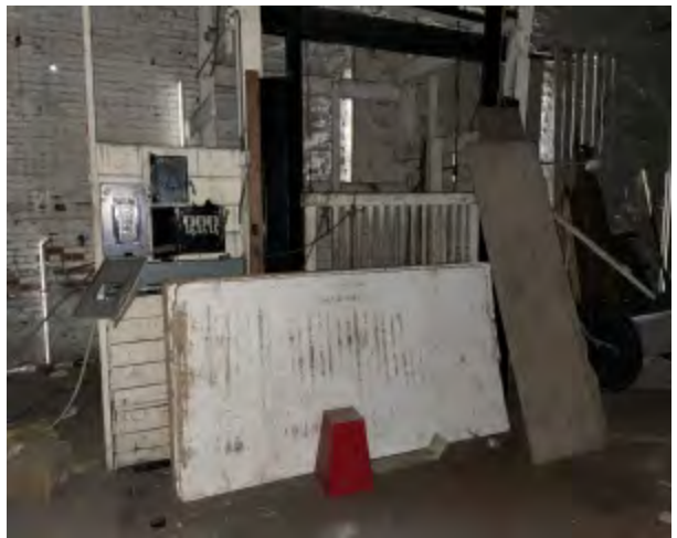
Photo 4 Comments: Elevator lift system located southeast of north corner of building.
