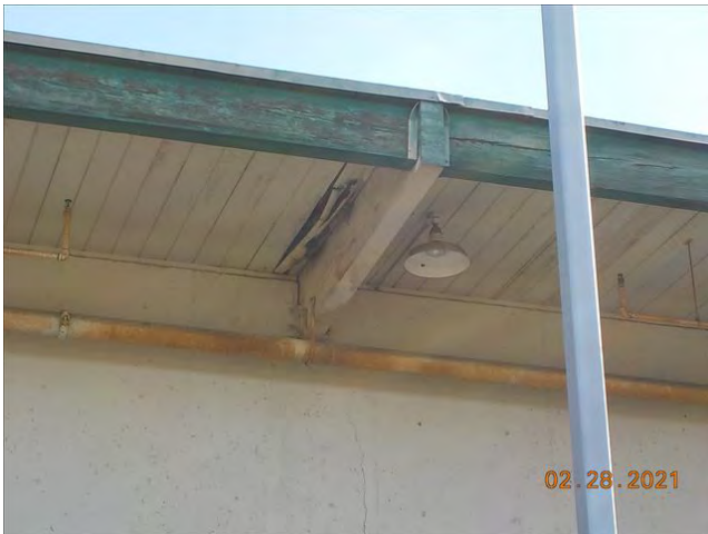
Date: 2/28/2021 9:36:35 AM DAMAGED ROOF ON PARKING LOT SIDE OF STRUCTURE
