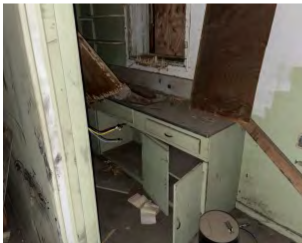
Photo 12 Comments: Small room near the south corner of the building containing a small kitchen like area.
