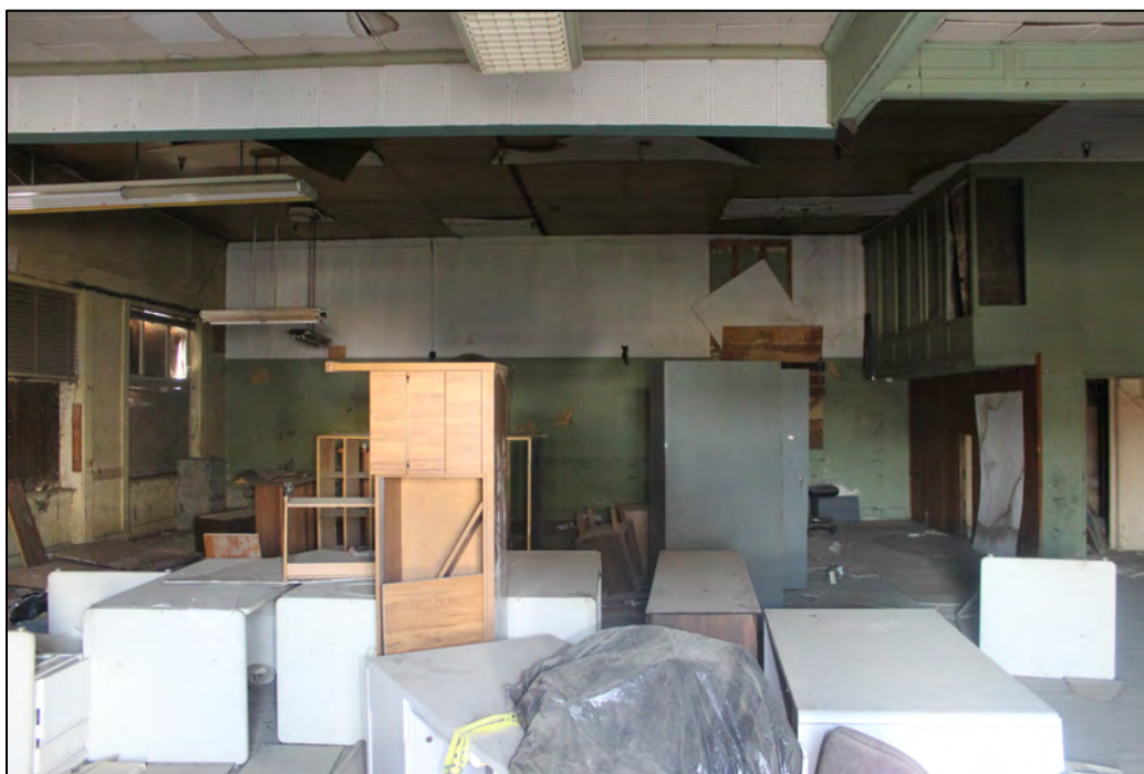
Photograph 11. Overview of former office area on the interior of 735, 739, and 741 H Street, camera facing west, October 13, 2022.
