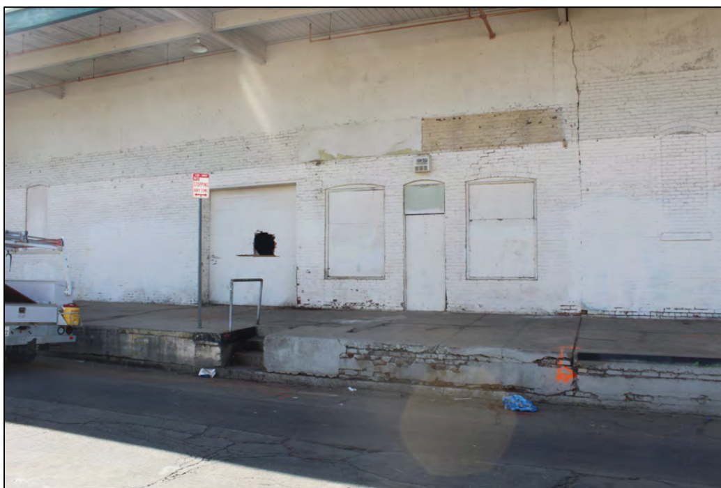
Photograph 5. View of brick loading dock and foundation, with exposed brick showing through the concrete and view of bricked over windows and entryways, camera facing west, October 13, 2022.
