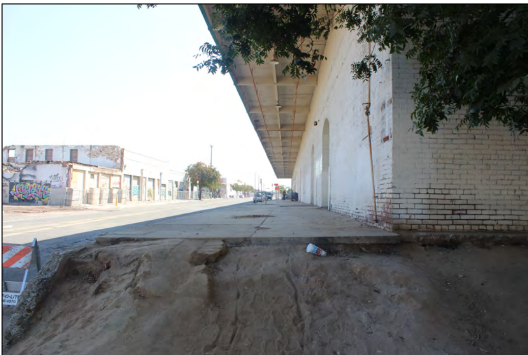
Photograph 7. View of where loading dock and former buildings were demolished and removed on north elevation of 735, 739, and 741 H Street, camera facing south, October 13, 2022.
