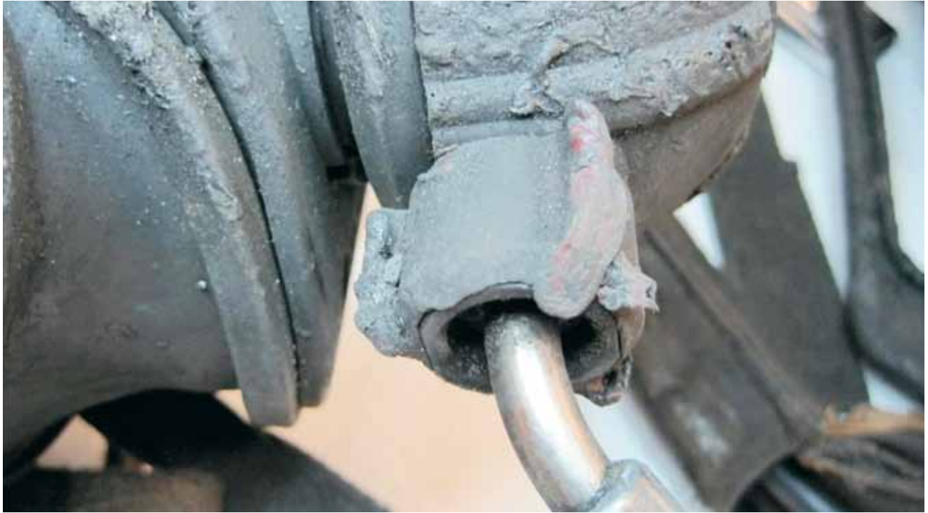
Figure 7: Melted bypass knob.
