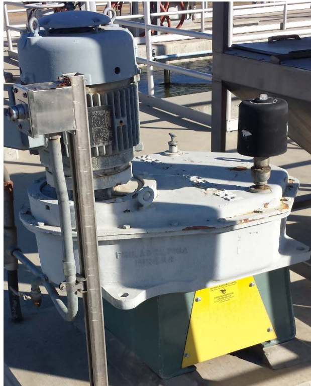
Figure 5.19: Injection Mixer Motor and Gear Box
