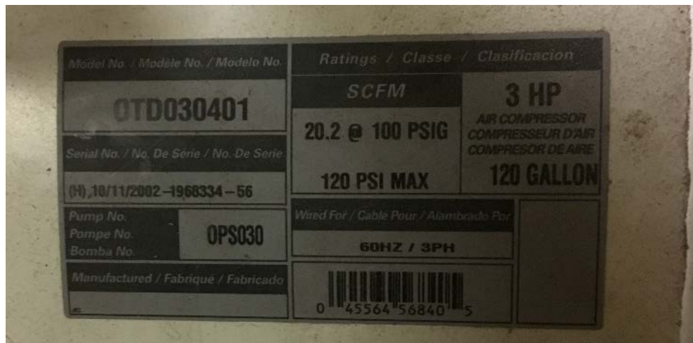
Figure 5.36: Air Compressor Nameplate
