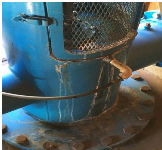
Figure 4.29: Corrosion at Booster Pump
