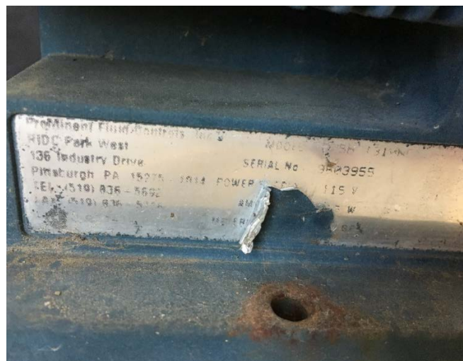
Figure 4.70: Orthopolyphosphate Pump Nameplate
