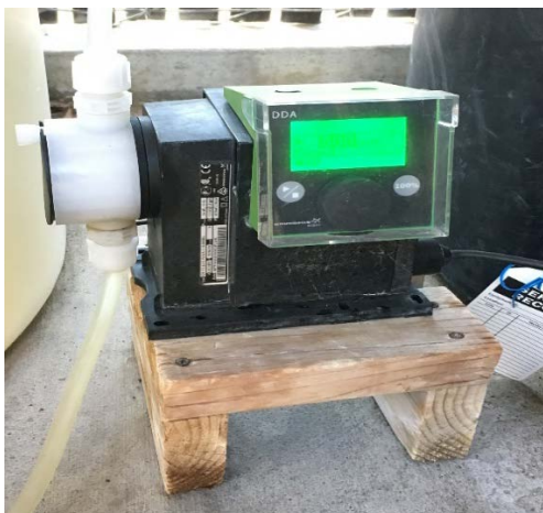
Figure 4.51: Chlorine Dosing Pump at Wellhead Site 70
