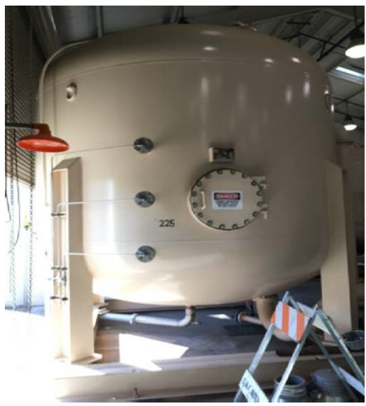
Figure 4.15: GAC Vessel at Wellhead Site 225
