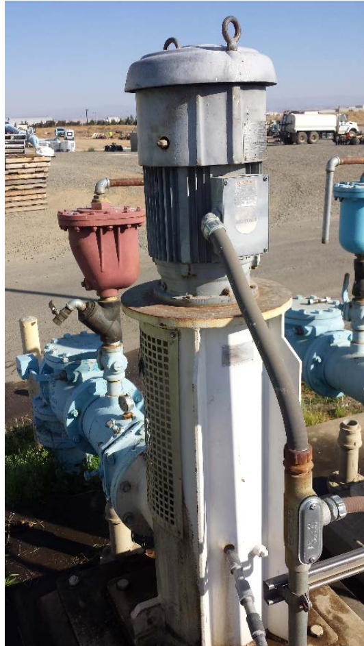
Figure 5.83: Oil Stains Around Washwater Pump and Motor
