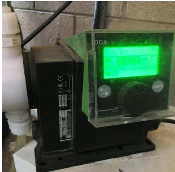
Figure 4.67: Post-Chlorine Dosing Pump at Wellhead Site 70
