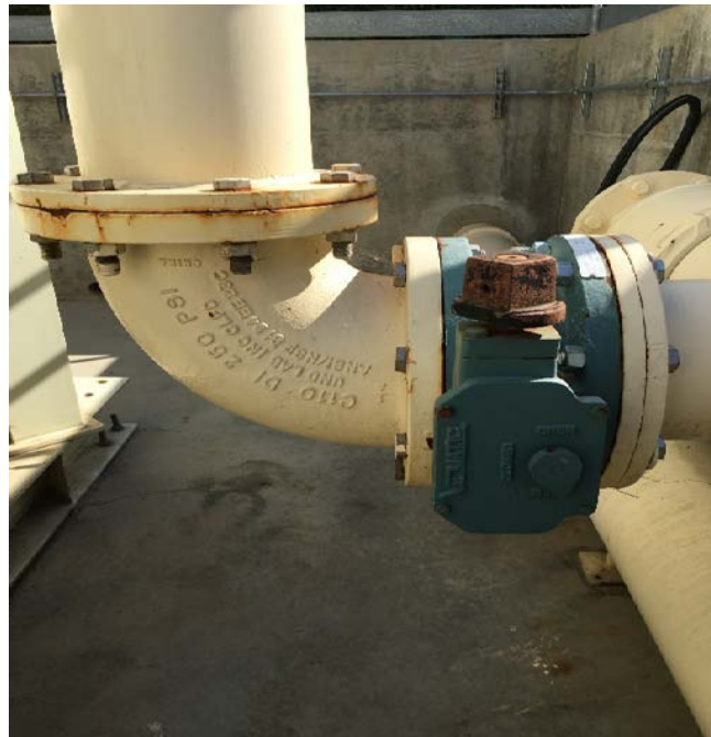
Figure 4.10: Minor Corrosion at GAC Vessel Piping Flanged Connections
