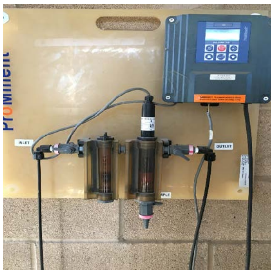
Figure 4.49: Chlorine Analyzing System at Wellhead Site 330
