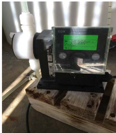
Figure 4.12: Chlorine Dosing Pump at Wellhead Site 354
