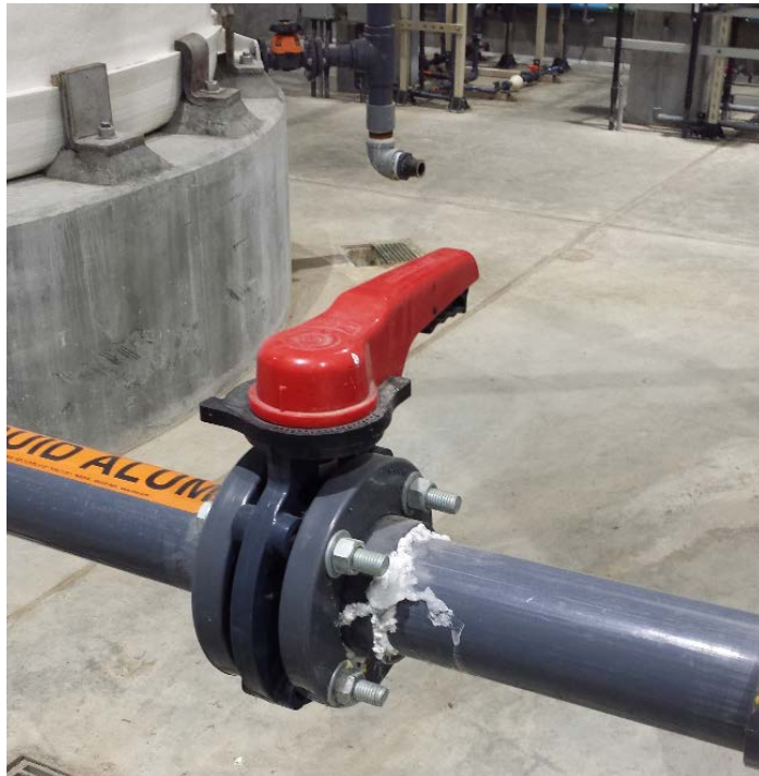
Figure 5.60: Build-up on Alum/Ferric Storage Piping
