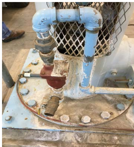
Figure 4.23: Corrosion at Boost Pump #1
