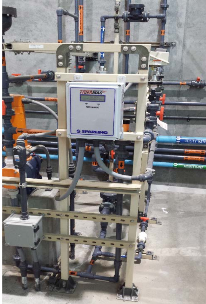
Figure 5.59: Cationic Polymer Feed Pump System
