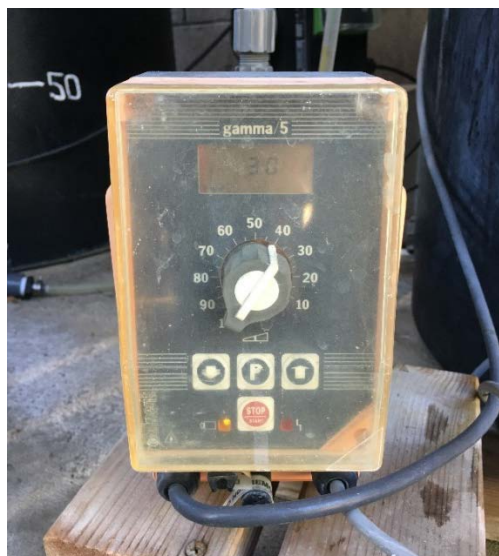
Figure 4.69: Orthopolyphosphate Dosing Pump at Wellhead Site 70
