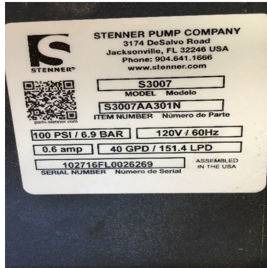
Figure 4.47: Chlorine Dosing Pump Nameplate
