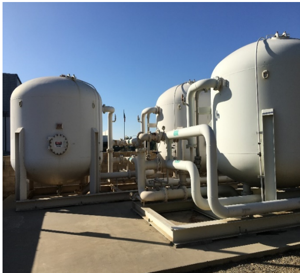
Figure 4.62: GAC Vessels at Wellhead Site 70
