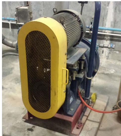
Figure 5.27: Solids Pump and Electric Motor
