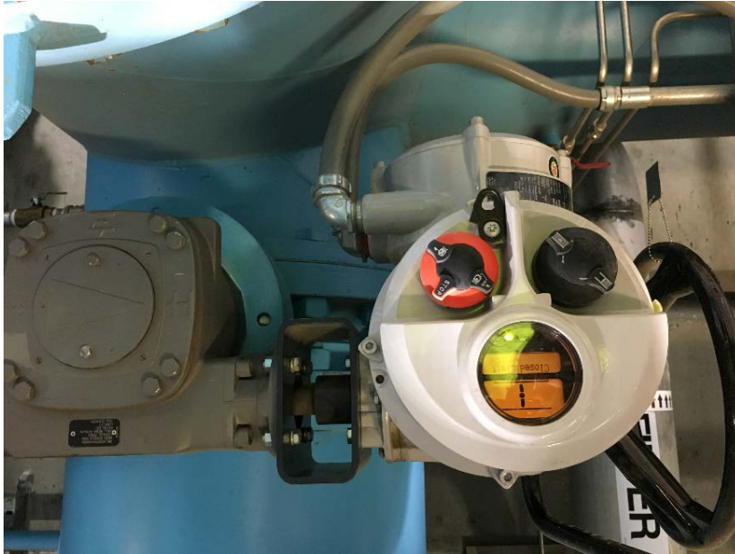
Figure 5.45: Backwash Valve and Actuator
