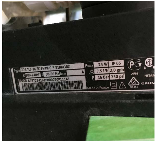
Figure 4.68: Post-Chlorination Pump Nameplate
