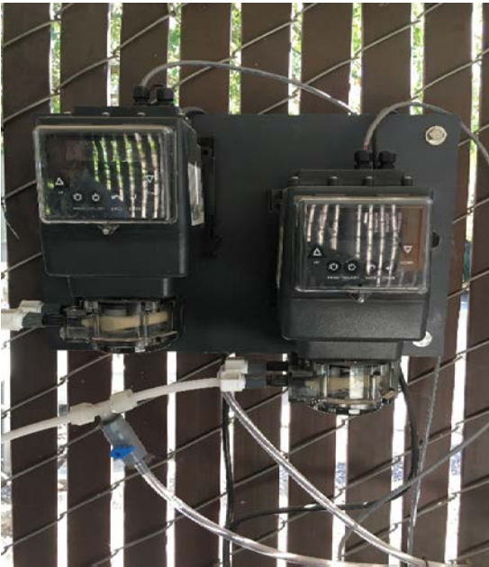
Figure 4.36: Chlorine & Orthopolyphosphate Dosing Pump at Wellhead Site 143
