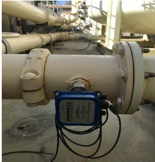
Figure 4.11: GAC Outlet Flow Meter No. 3
