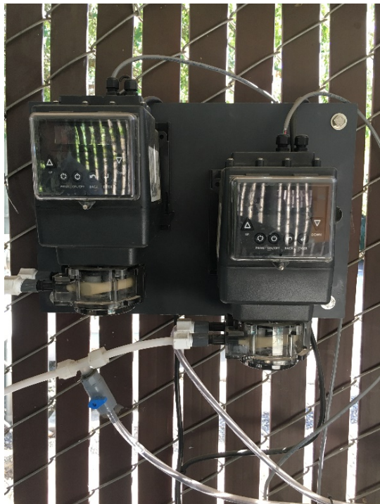
Figure 4.34: Chlorine & Dosing Pump at Wellhead Site 143
