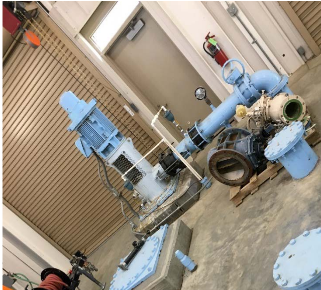
Figure 4.21: Booster Pump #1 at Wellhead Site 225
