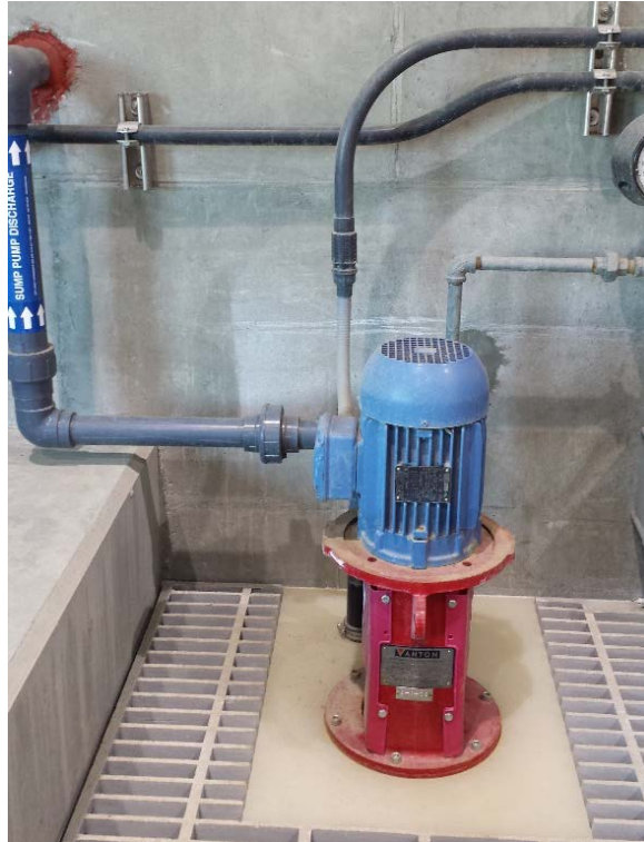
Figure 5.77: Typical Chemical Sump Pump
