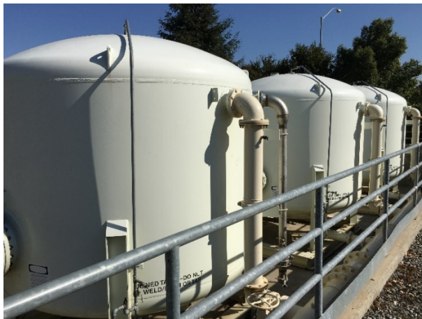
Figure 4.8: GAC Vessels at Wellhead Site 354
