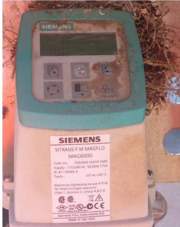
Figure 5.11: Flow Meter Control panel
