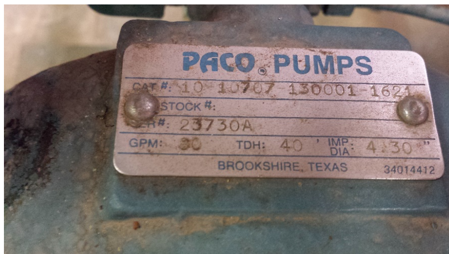
Figure 5.78: Potable Water Booster Pump Nameplate
