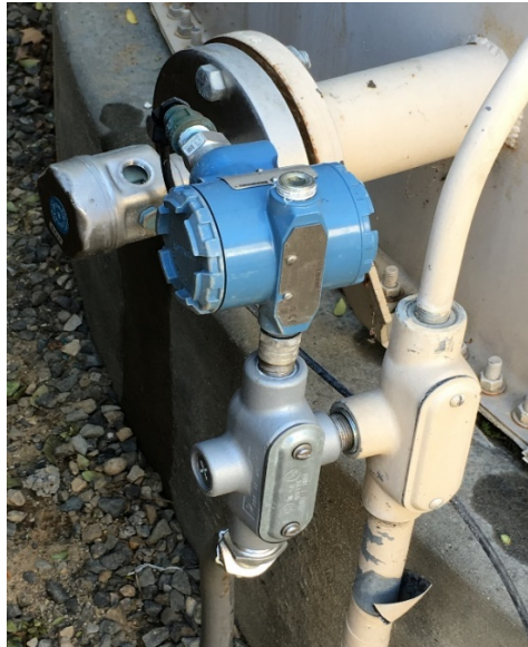
Figure 4.30: Degassing Tank Level Instrument at Wellhead Site 143
