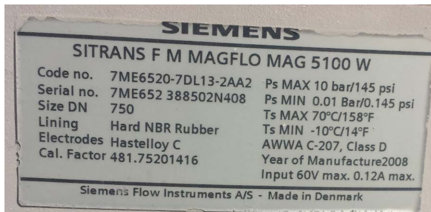
Figure 5.10: Flow Meter Nameplate
