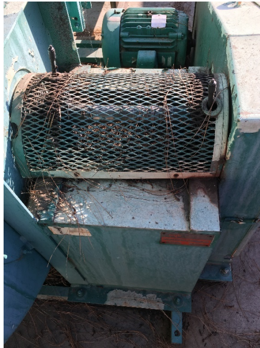
Figure 4.56: Corrosion and Chipping Paint at Air Blower
