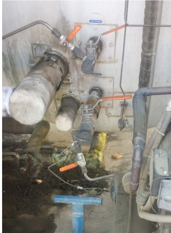
Figure 5.73: Carbon Dioxide Tank Instruments and Equipment
