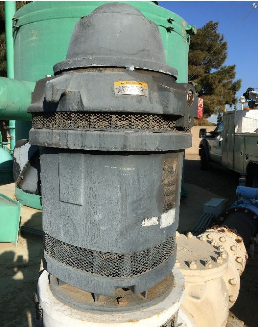
Figure 4.59: Minor Corrosion of Motor
