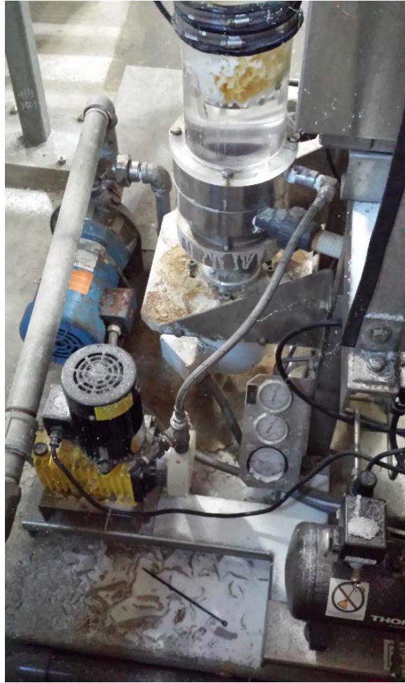
Figure 5.57: Polymer Batching System
