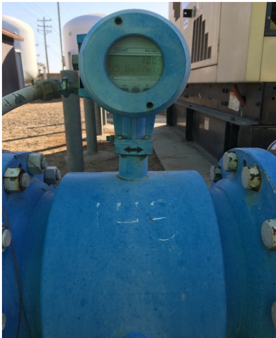
Figure 4.60: Flow Meter No. 1 at Wellhead Site 70
