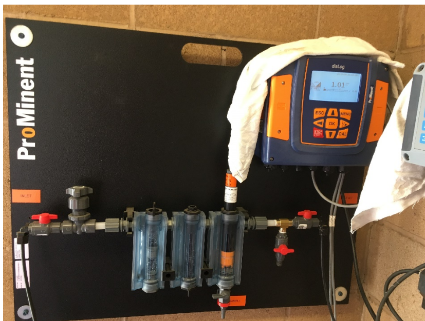
Figure 4.14: Chlorine Analyzing System at Wellhead Site 354
