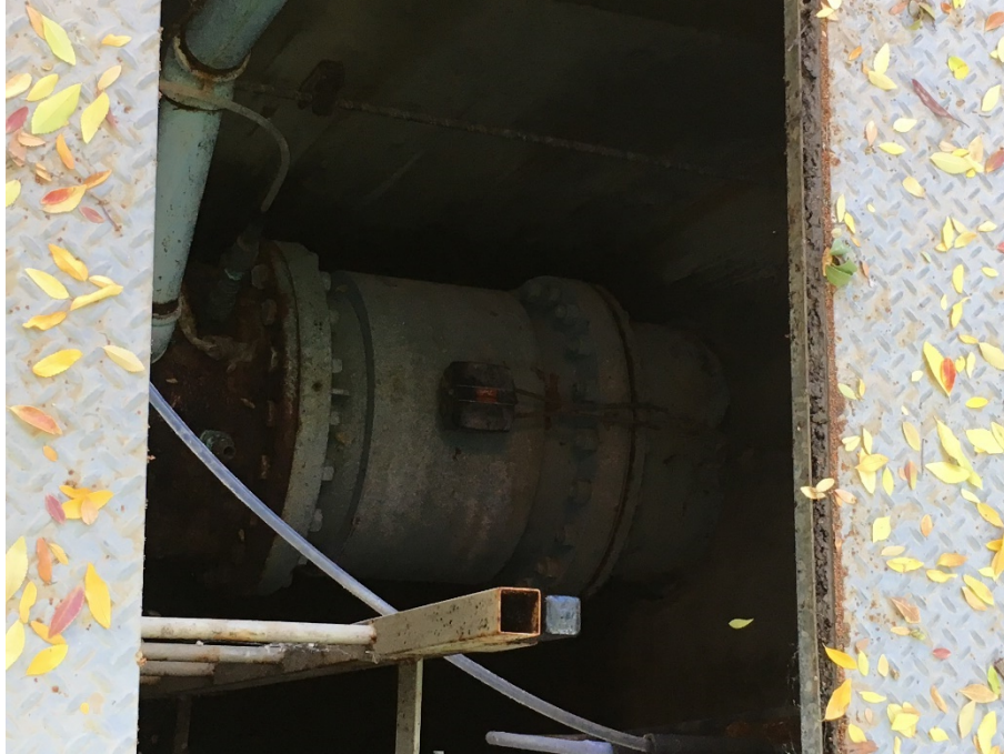
Figure 4.26: Flow Meter No. 2 at Wellhead Site 225
