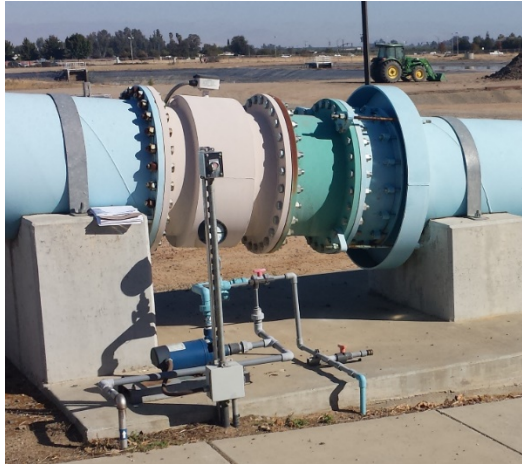
Figure 5.9: Plant Influent Flow Meter
