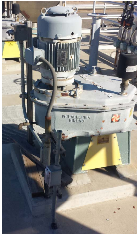
Figure 5.16: Coagulation Mixer Electric Motor and Gear box
