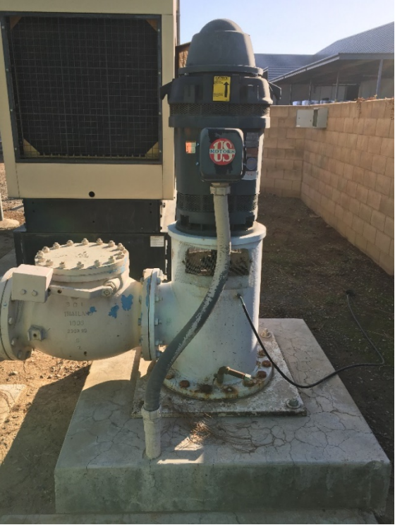
Figure 4.57: Booster Pump at Wellhead Site 70
