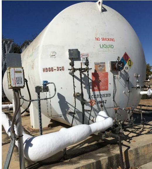
Figure 5.33: LOX Storage Tank with Ice Build-up on the Pipe
