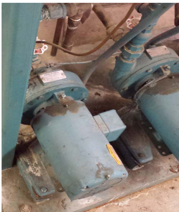
Figure 5.79: Potable Water Booster Pump
