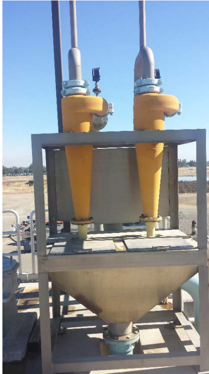
Figure 5.25: Hydrocyclones at Actiflo No. 1
