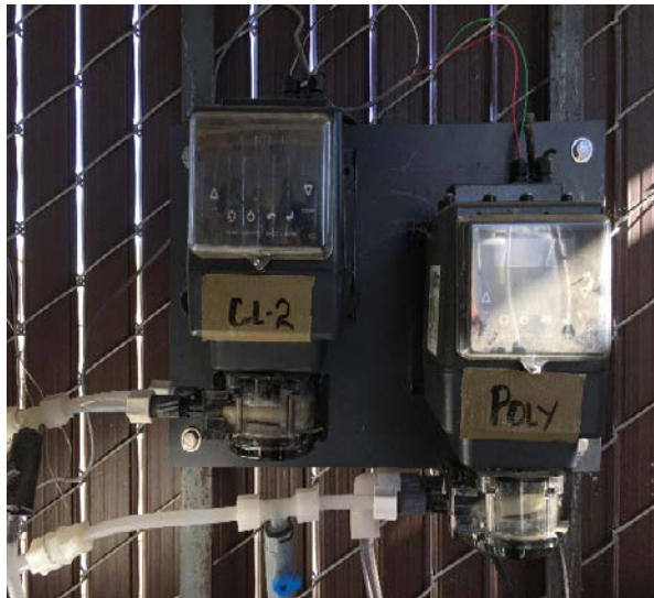
Figure 4.46: Chlorine & Orthopolyphosphate Dosing Pump
