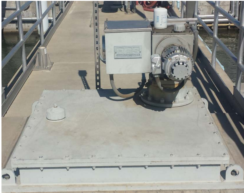
Figure 5.24: Sludge Scraper Electric Components at the Clarifier Deck
