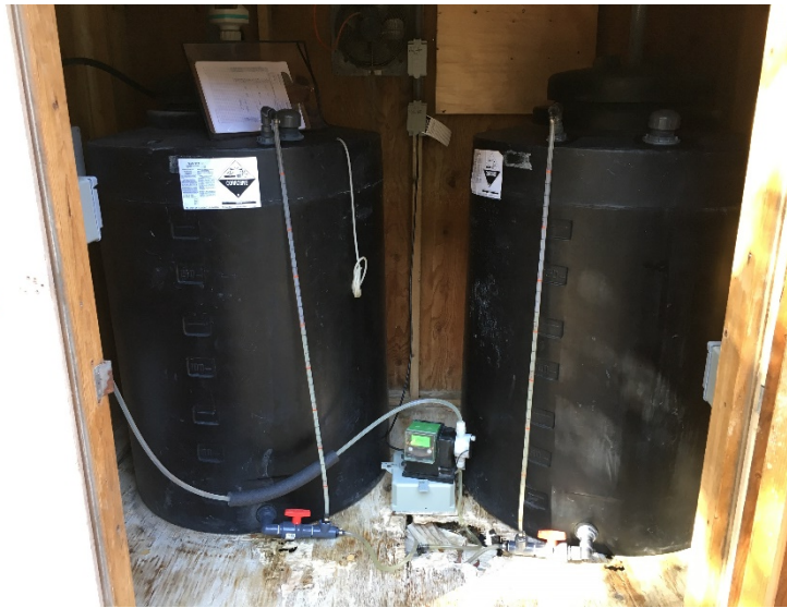
Figure 4.20: Sodium Hypochlorite Tank and Pump at Wellhead Site 225
