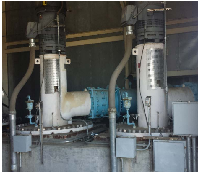
Figure 5.51: Backwash Supply Pumps
