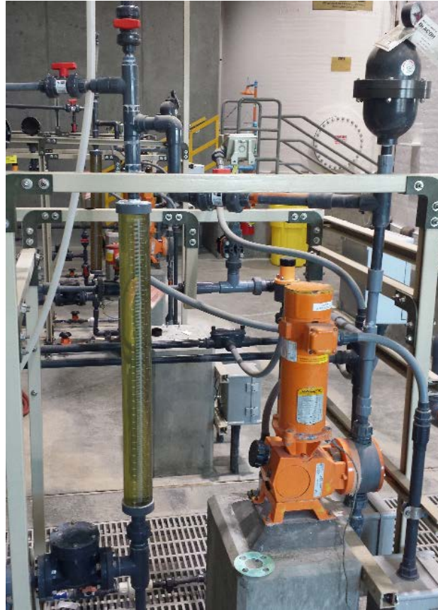
Figure 5.56: Sodium Hypochlorite Feed Pump
