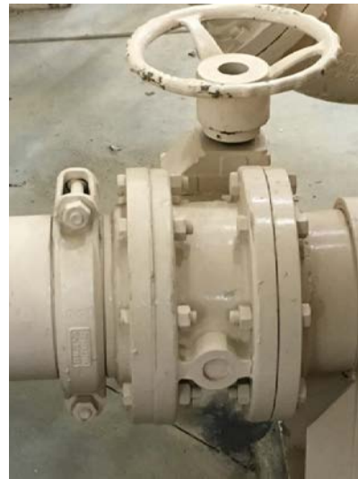
Figure 4.25: Well 225 Effluent Control Valve
