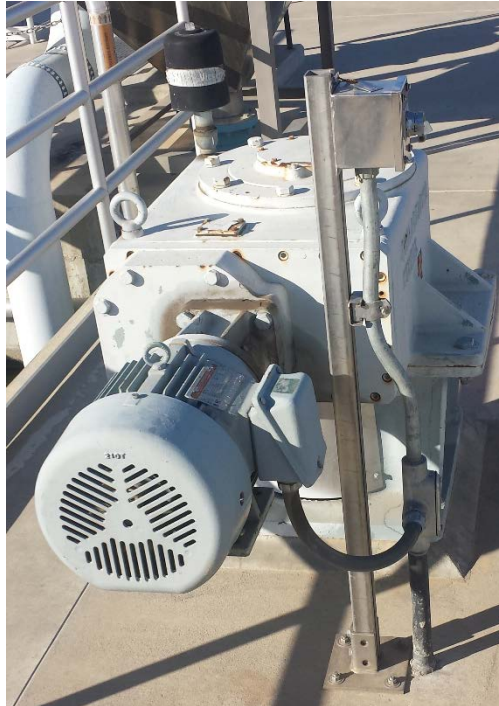
Figure 5.22: Flocculation Mixer Electrical Components at Clarifier Deck
