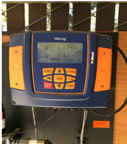
Figure 4.40: pH Analyzer at Wellhead Site 143
