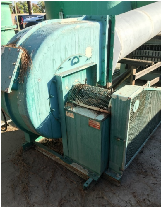
Figure 4.54: Air Blower at Wellhead Site 70
