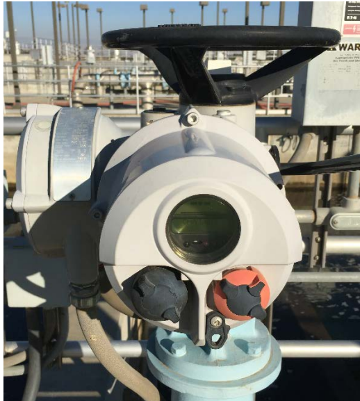
Figure 5.43: Influent Valve Actuator
