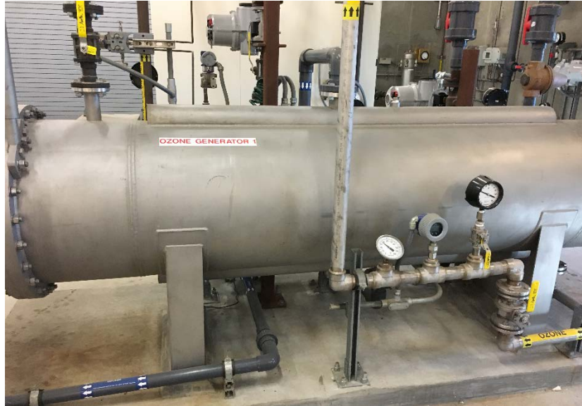
Figure 5.40: Ozone Generator Unit No. 1
