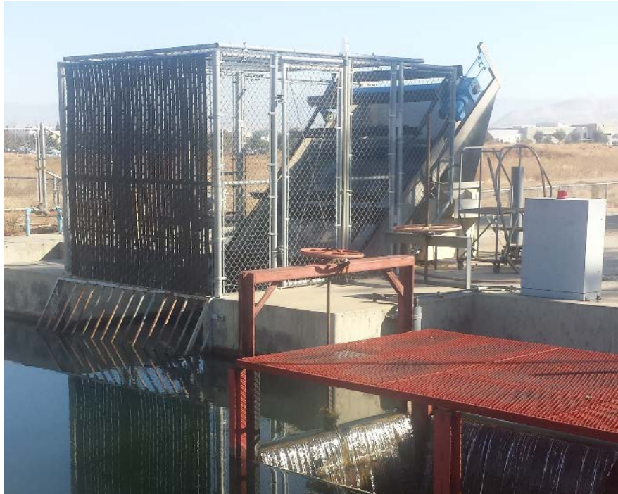
Figure 5.2: General View of Water Inlet Process
