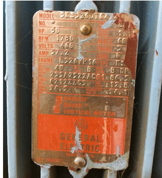
Figure 4.22: Booster Pump Motor #1 Nameplate
