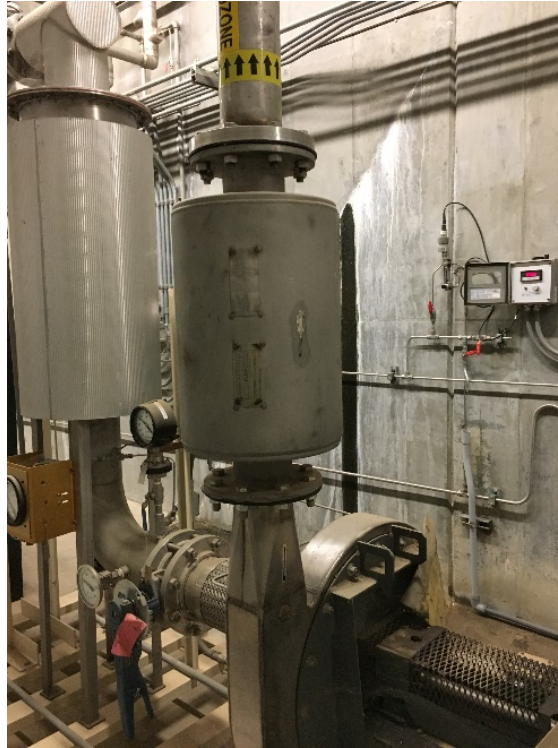
Figure 5.41: Ozone Destruct Unit No. 1
