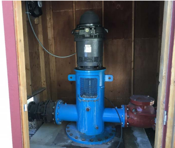
Figure 4.28: Booster Pump and Motor at Wellhead Site 143
