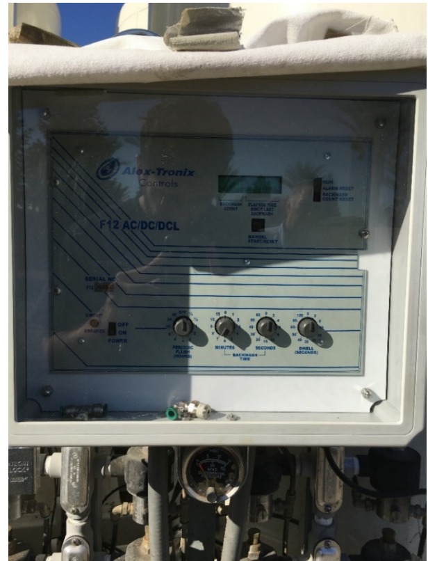
Figure 4.45: Filter Control Panel
