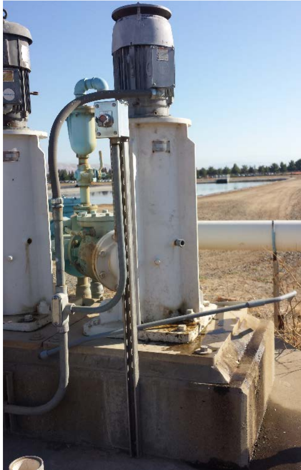
Figure 5.85: Decant Pump 7-P-31 and Electric Motor
