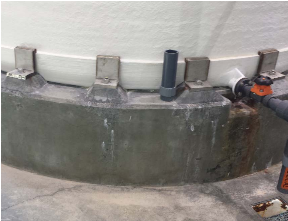
Figure 5.54: Leaking at Sodium Hypochlorite Tank Flanged Connection
