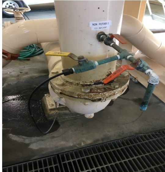
Figure 4.17: Corrosion at GAC Vessel Outlet Piping
