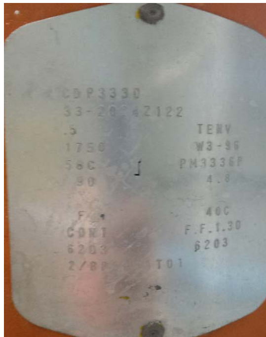
Figure 5.70: Polyphosphate Pump Motor Nameplate
