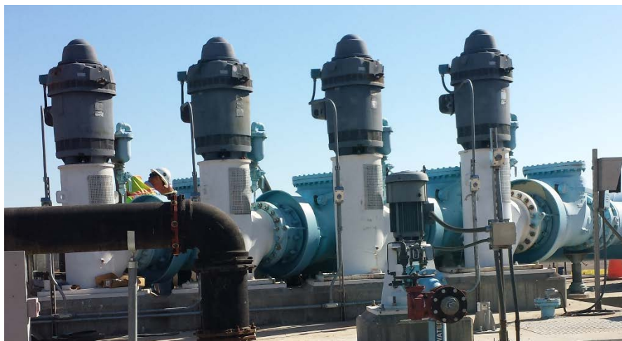
Figure 5.7: Raw Water Pumps
