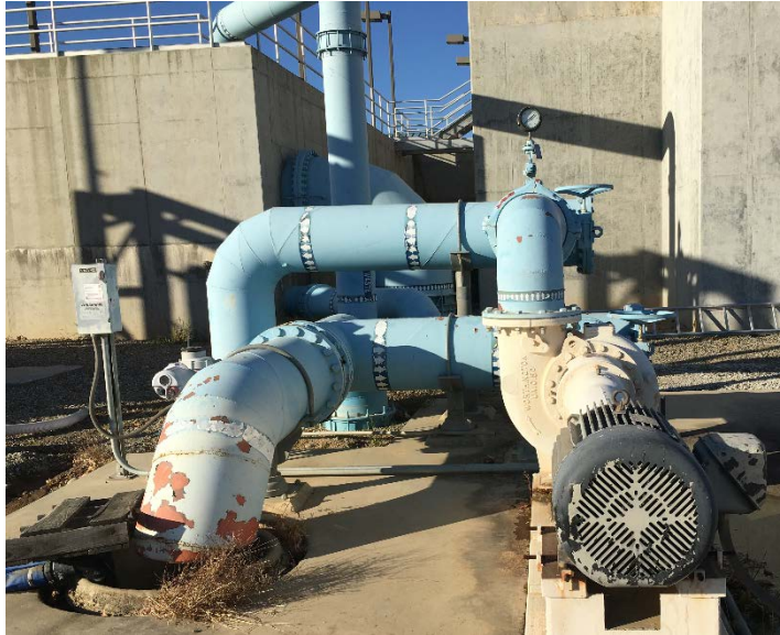
Figure 5.48: Filter Waste Pump Actuator and Valve
