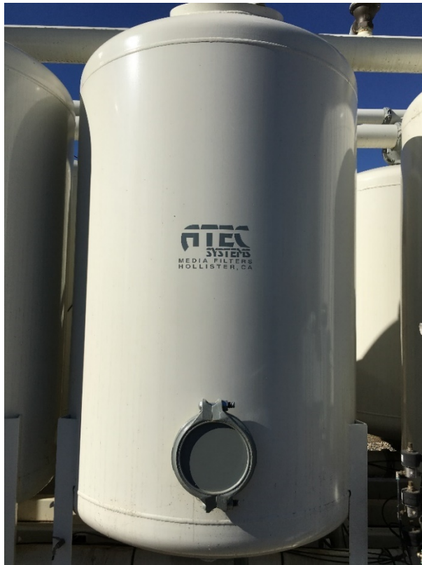
Figure 4.44: Filter Vessel at Wellhead Site 143
