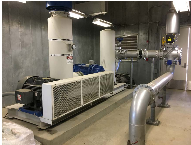
Figure 5.50: Air Scour Blower
