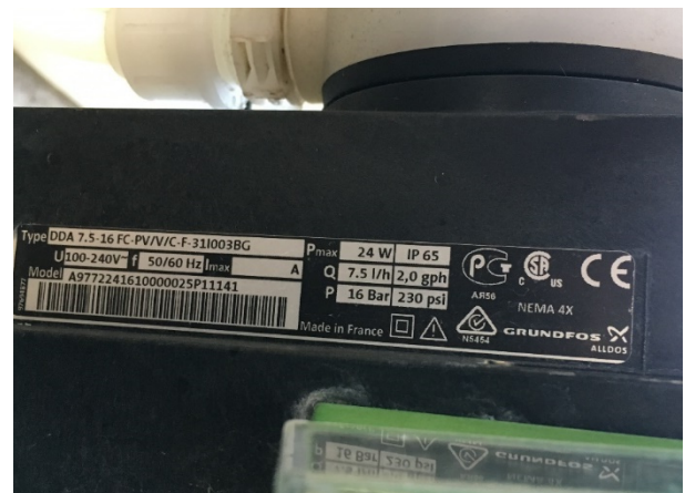
Figure 4.52: Pre-Chlorination Pump Nameplate
