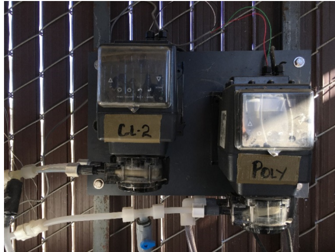
Figure 4.48: Chlorine & Orthopolyphosphate Dosing Pump
