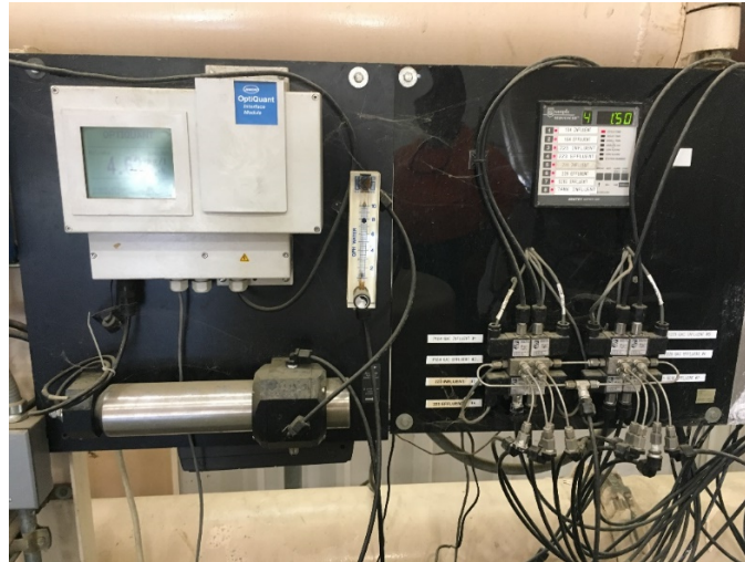
Figure 4.18: Nitrate Analyzing System at Wellhead Site 225
