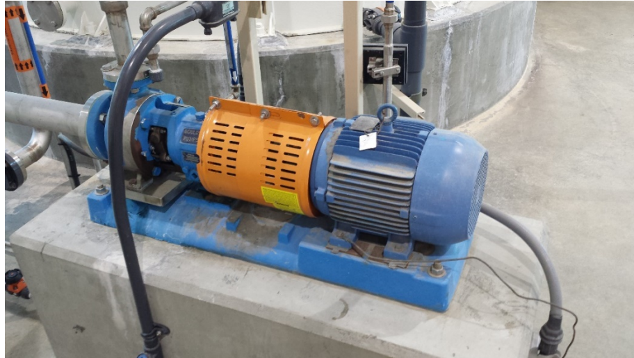
Figure 5.68: Caustic System Mixing Pump
