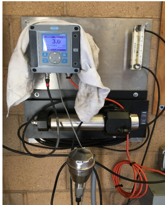
Figure 4.13: Nitrate Analyzer at Wellhead Site 354
