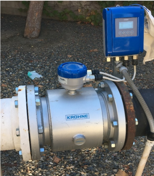
Figure 4.32: Flow Meter No. 1 at Wellhead Site 143
