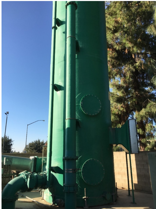
Figure 4.53: Packed Tower at Well 70
