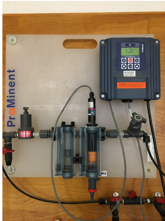
Figure 4.19: Chlorine Analyzing System at Wellhead Site 225
