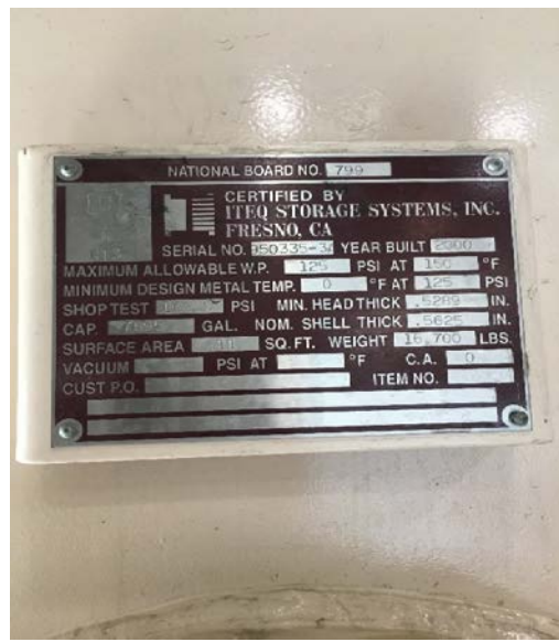
Figure 4.16: GAC Vessel Nameplate at Wellhead Site 225
