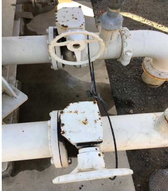
Figure 4.64: Oil and Minor Corrosion at Valve Housings
