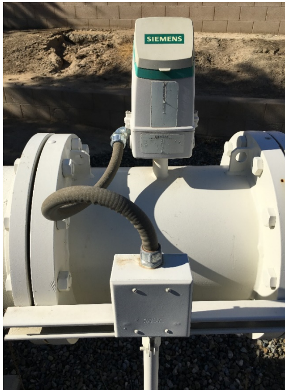
Figure 4.42: Flow Meter No. 1 at Wellhead Site 330
