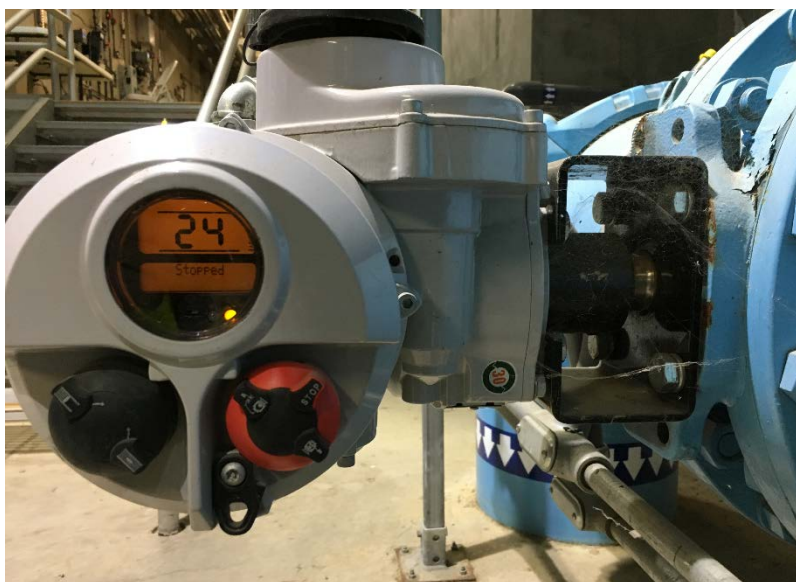
Figure 5.44: Filter Water Valve and Actuator
