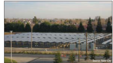
SOLAR ARRAYS. Yuba City has entered a public-private partnership to build a 770-kilowatt solar photovoltaic array in a stormwater detention basins, sharing space efficiently and supplying energy at low cost to the city.
