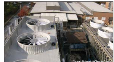
COGENERATION. Combined heat and power technologies are used widely in institutional settings, such as college campuses. Cogeneration is also applied around the world in residential and mixed-use settings.
